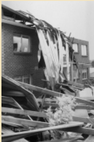
Storm Brisbane, Qld 1985 Major damage to a range of infrastrucrure was sustained during this extreme event
