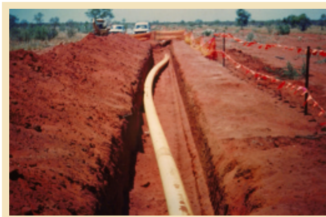
Gas Pipeline Tennant Creek Earthquake 1988 The pipeline which supplied Darwin's electricity system was damaged during this Earthquake.
